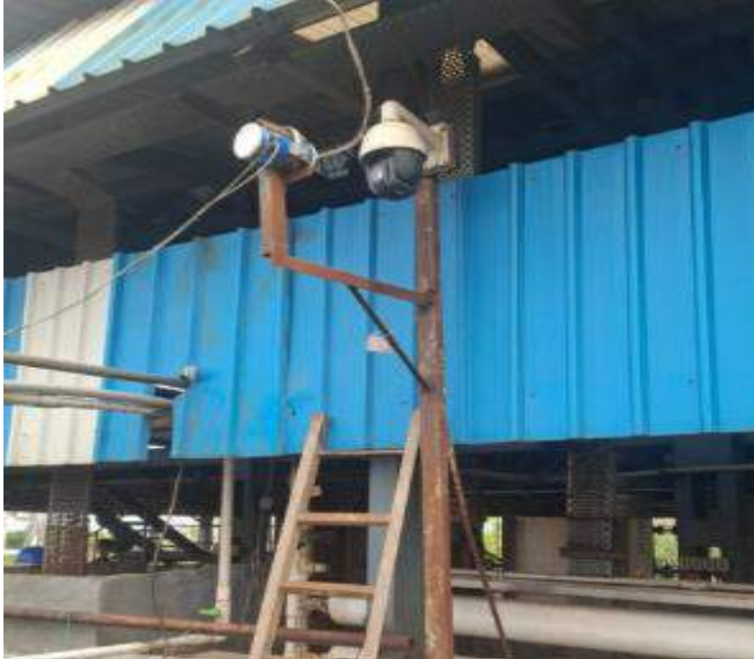
CEMS SYSTEM CAMERA AND FLOW METER
